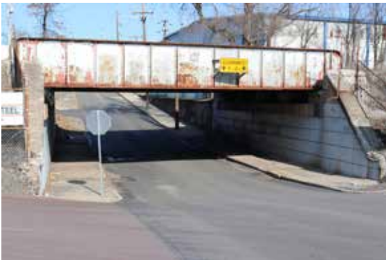
The clearance of this Norfolk Southern rail bridge is too low for most large trucks and tractor trailers to pass under, forcing most traffic to return from Industrial Highway.
